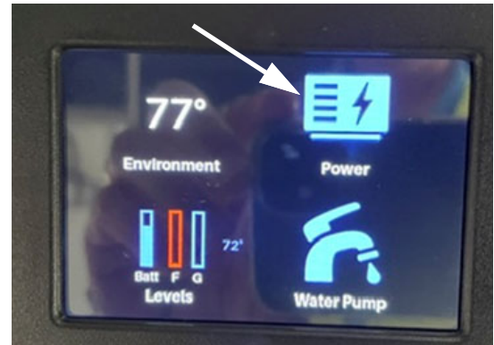
Power icon. -Typical View
