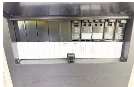
120-Volt Circuit Breakers -Typical View
