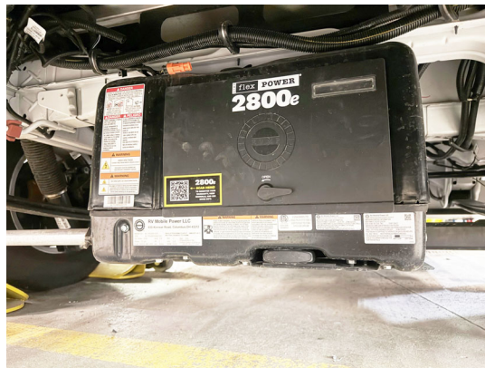
4. The generator is located underneath the rear end of the motorhome. -Typical View
