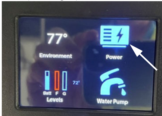
1. Generator location on the main screen of the Systems Monitor Panel -Typical View
