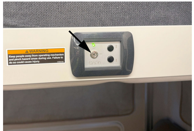
3. Turn the key (located near the monitor panel) to the “ON” position. -Typical View
