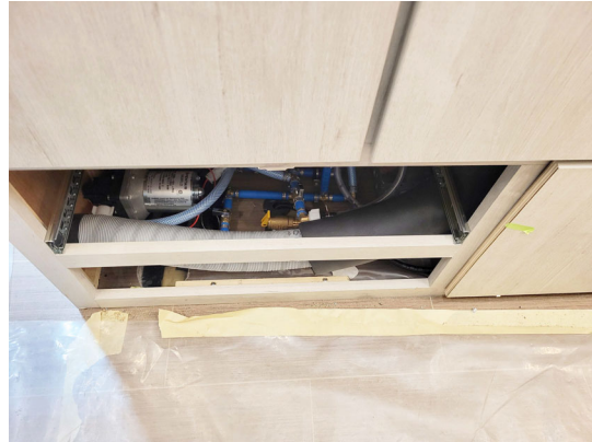
Water Pump Access Panel (Located under the galley. To access remove bottom drawer.) -Typical View
