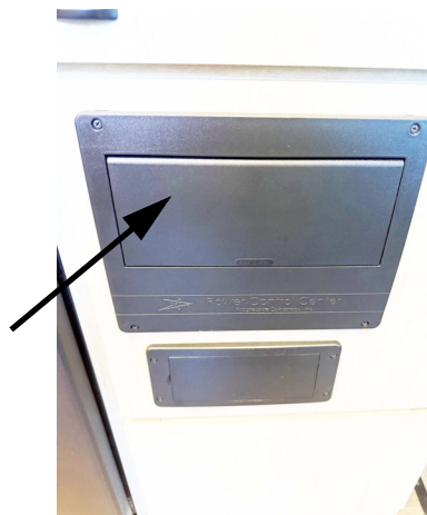
The breaker box is located above the fuse box on the inside wall. -Typical View
