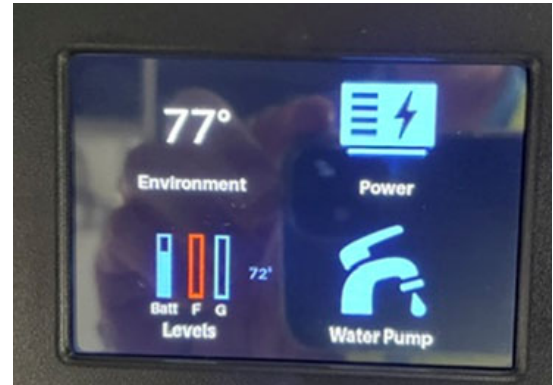
System Monitor Panel -Typical View
