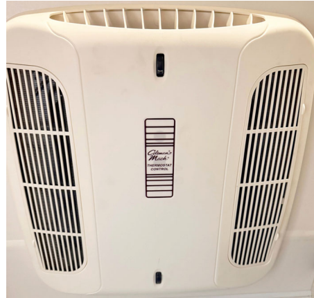
Air conditioner vent located on the ceiling of the motorhome. -Typical View
