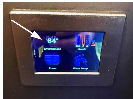
Climate control on the System Monitor Panel -Typical View
