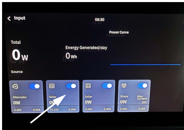
Solar Charge Controls (Located on the EcoFlow monitor panel) -Typical View
