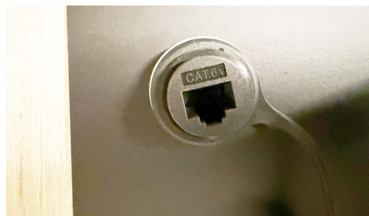
Ethernet hook up for satellite located inside the coach in the overhead cabinet above the refrigerator. -Typical View
